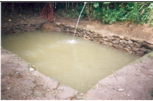
Water Harvesting Tank on Hill Slopes
