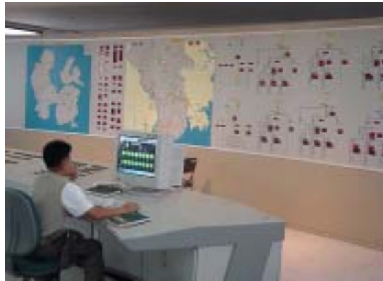
Figure 6 TM/TC control center
